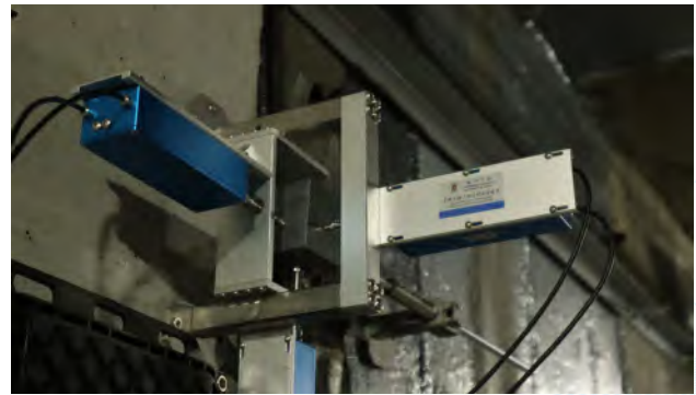
光纖光柵傳感器安裝在港珠澳大橋沉管隧道 Fibre grating sensors installed in the immersed tube tunnel of the HZMB
