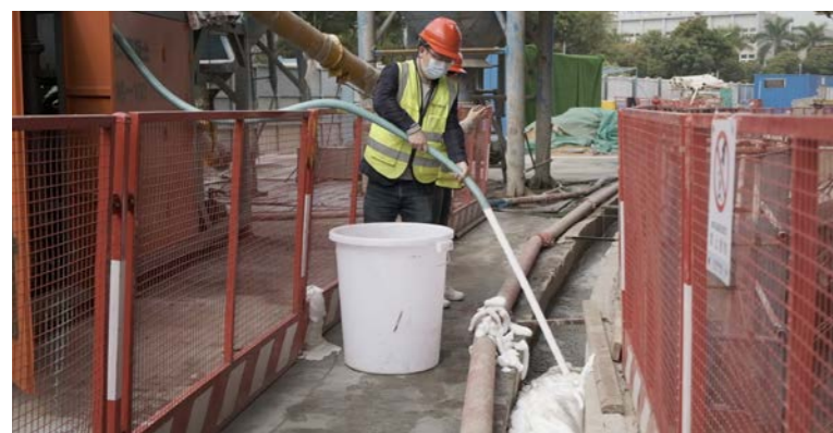
納米泡沫混凝土技術應用於珠海高新技術產業開發區的實際工程 UM's construction technique using nano-foam concrete is applied in the Zhuhai National Hi-tech Industrial Development Zone
